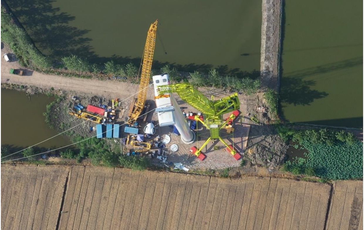
Vestas 3.3mw-137m Wind Farm in Jiangsu ZhouShan
