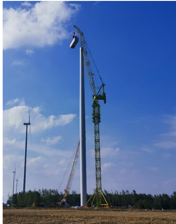
Vestas 3.3mw-137m Wind Farm in Jiangsu ZhouShan
