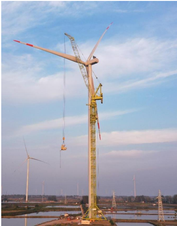
Vestas 3.3mw-142m Wind Farm in Jiangsu LongQiu
