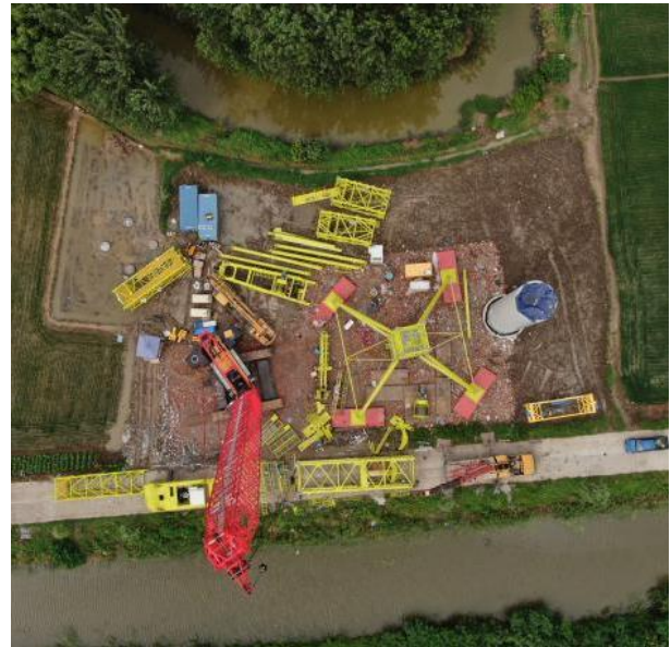
Vestas 3.3mw-152m Wind Farm in Jiangsu Xianfeng
