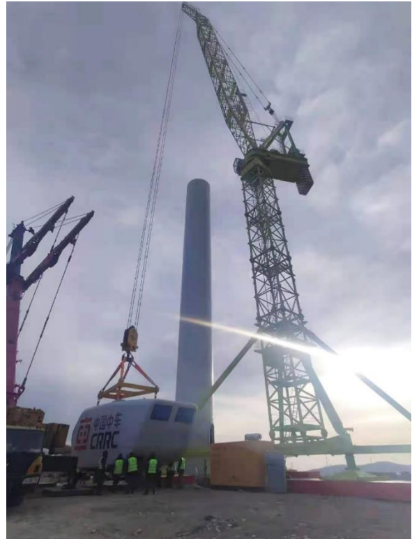
2.0mw-95m Mountain Wind Farm in Shanxi
