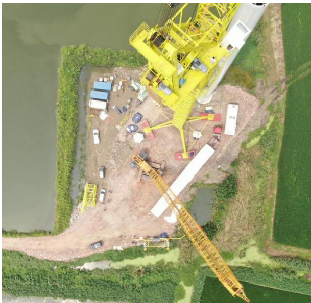
Vestas 3.3mw-142m Wind Farm in Jiangsu Longqiu
