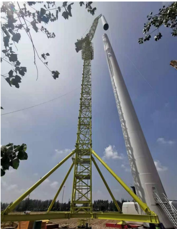
Vestas 3.3mw-152m Wind Farm in Jiangsu Xianfeng
