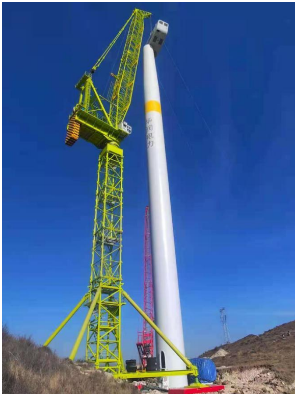
2.0mw-95m Mountain Wind Farm in Shanxi
